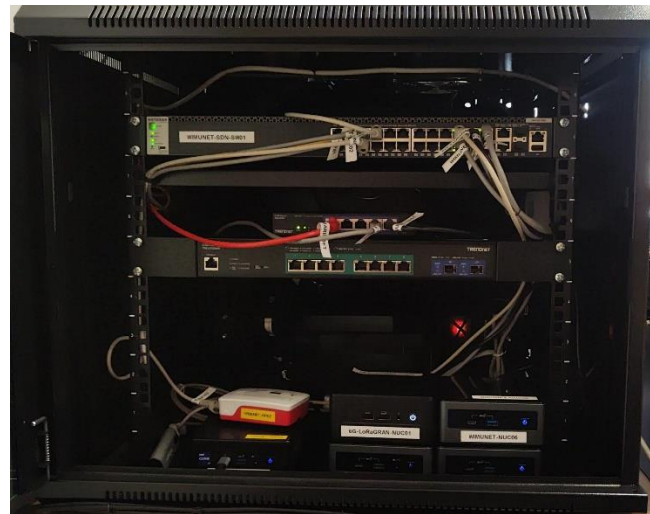
Figure 5. Rack cabinet with 6G-LoRaGRAN cluster.
