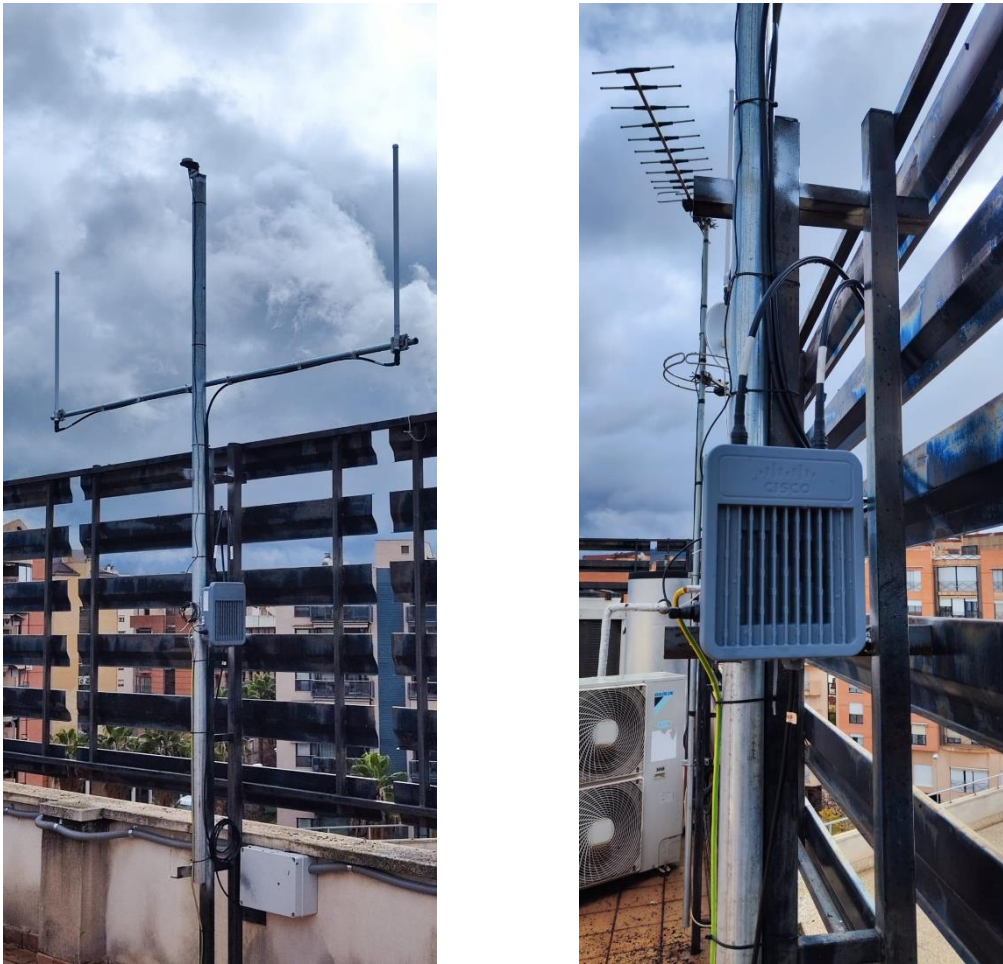
Figure 2. CISCO gateway at the roof of ETSIIT-UGR.
